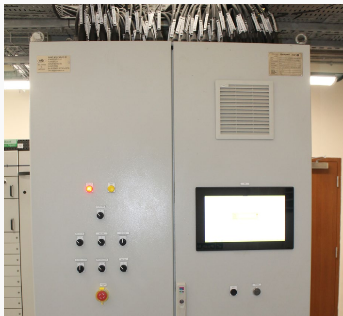
HVAC Control Panel Termination
