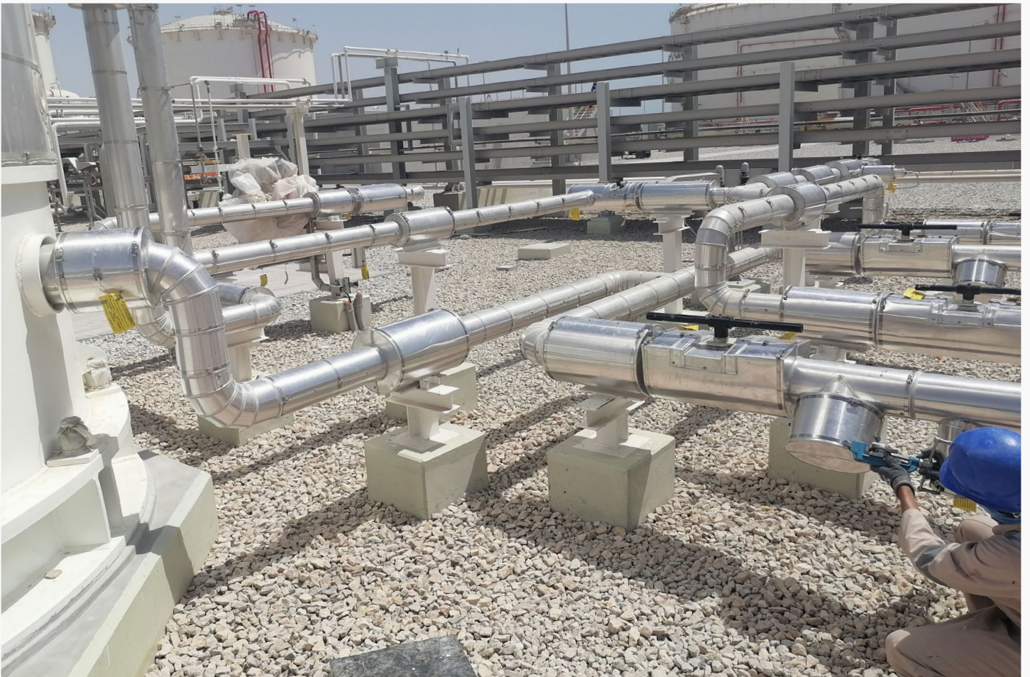
Insulation For Pipeline And Equipments
