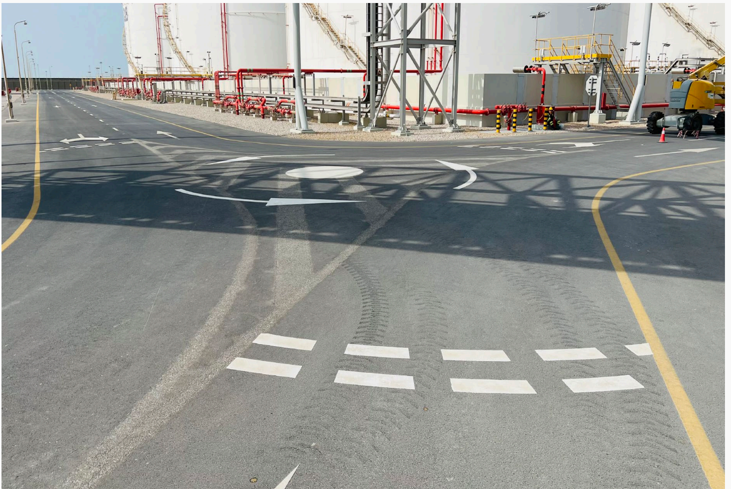
Construction Of Asphalt And Concrete Road Including Road Marking, Safety Sign Installation
