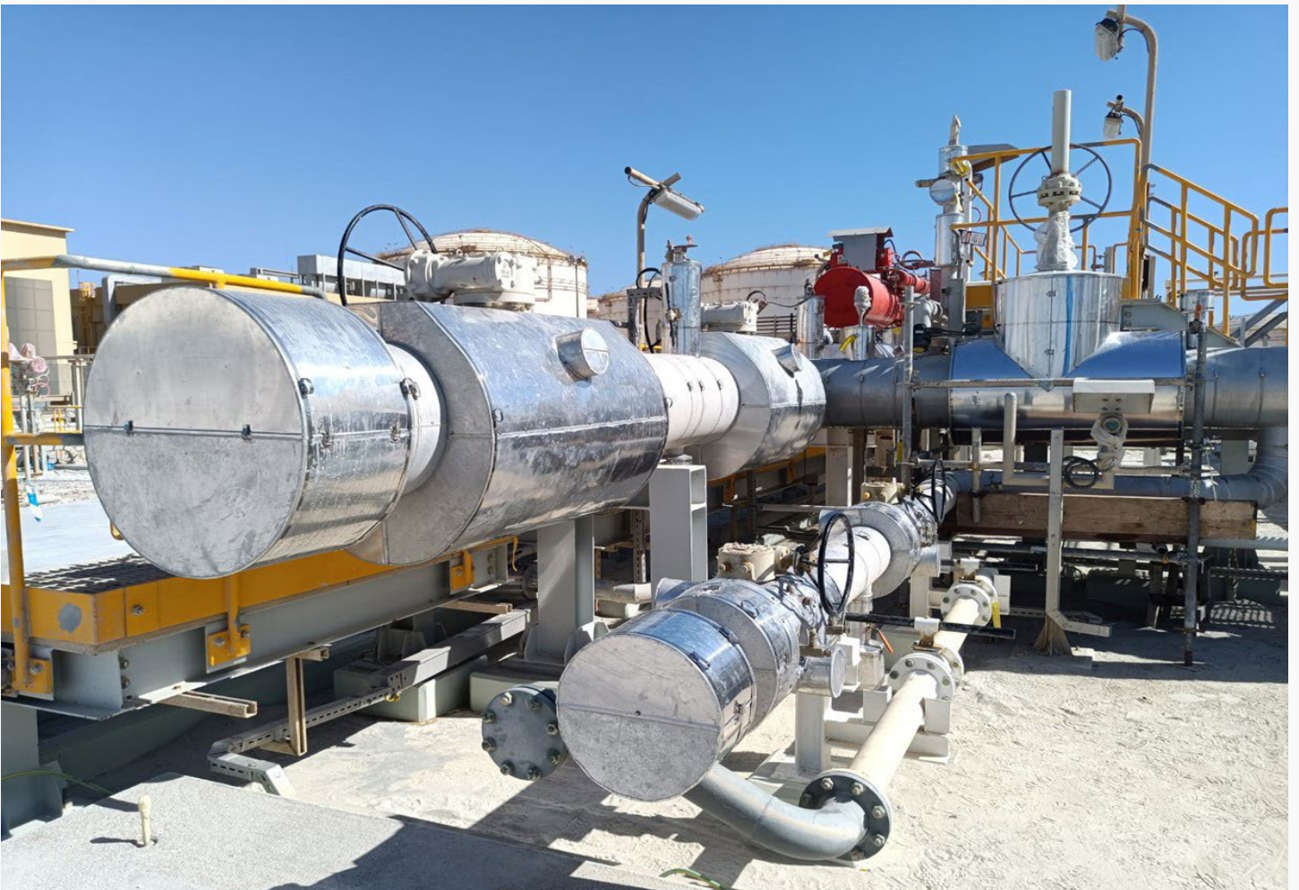
Insulation For Pipeline And Equipments
