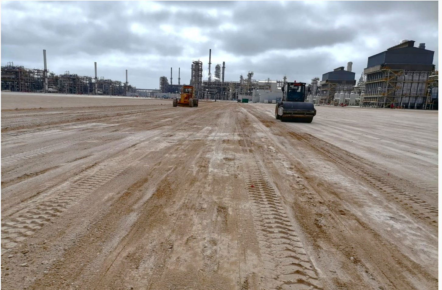
Leveling, Grading & Compaction Work For Oil And Gas, Power Plant And Petrochemical Plant
